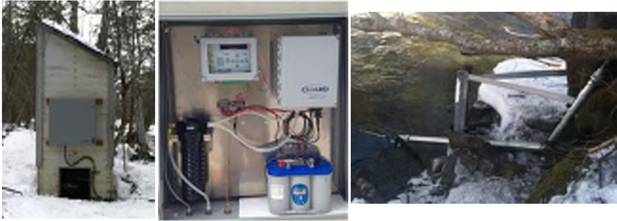
Figure 5. Monitoring equipment at Station ISF-2.
